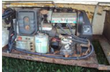
3.5K Kohler GenSet
