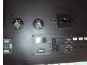
Disconnect / Genset Control
