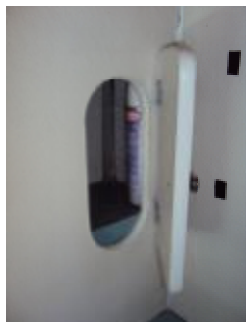
Sink with electrically controlled water supply
