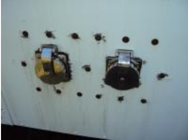
Shore Power Connections
